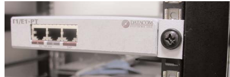
T1/E1-PT fastened on the right side of the equipment rack
